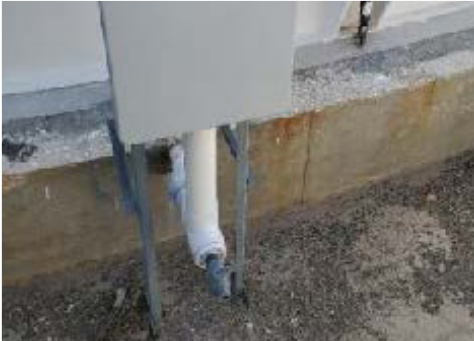
1. INSTALLED ER PROBE WITH ENCLOSURE
