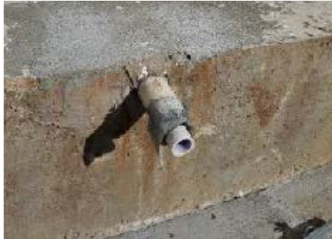
2. PREVIOUSLY INSTALLED COUPON PORT
