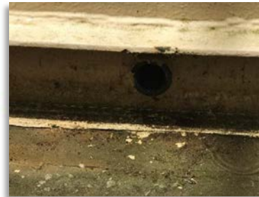
Dead Shell with Leak Port
