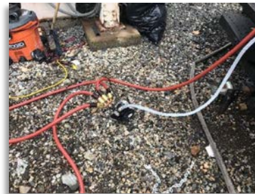
Pump for Injection
