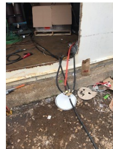
FIGURE 5: GARDEN HOSE MANIFOLD
