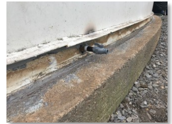
FIGURE 2: DEAD SHELL WITH LEAK PORT
