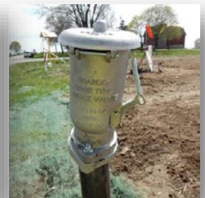
Pressure Release Valve
