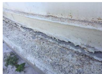
3. CHIME PLATE CONDITION
