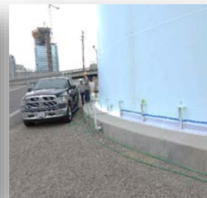
Inhibitor Injection Lines
