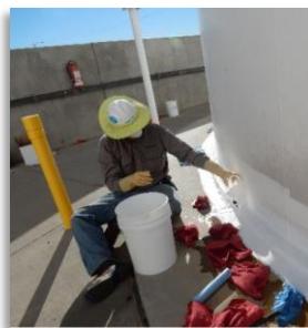
Inhibitor injection slurry.
