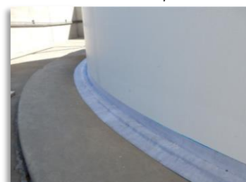
After the 2 nd coat of blue primer is the application of Viscotag EZ Wrap
