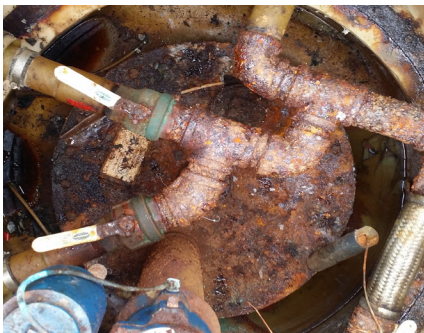
Sump corrosion caused by Ethanol and Acidic Vapor.
