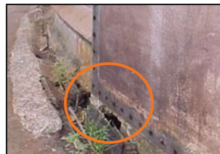
CORROSION HOLES IN THE AST BOTTOM
