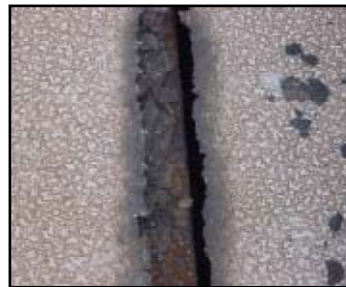
CORROSION AT A SUPPORT BEAM
