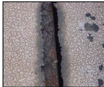
CORROSION AT A SUPPORT BEAM
