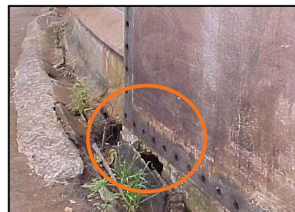
CORROSION HOLES IN THE AST BOTTOM
